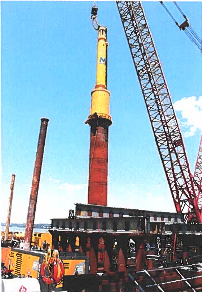
Trevcon brought in 60-ton hammers from Singapore for the Tappan Zee Test Pile Program.
